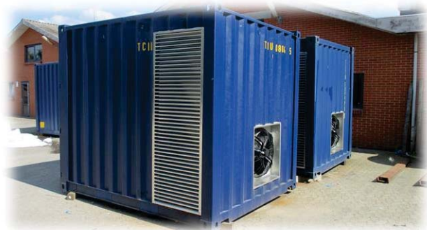
Complete ice plant, Container solution
